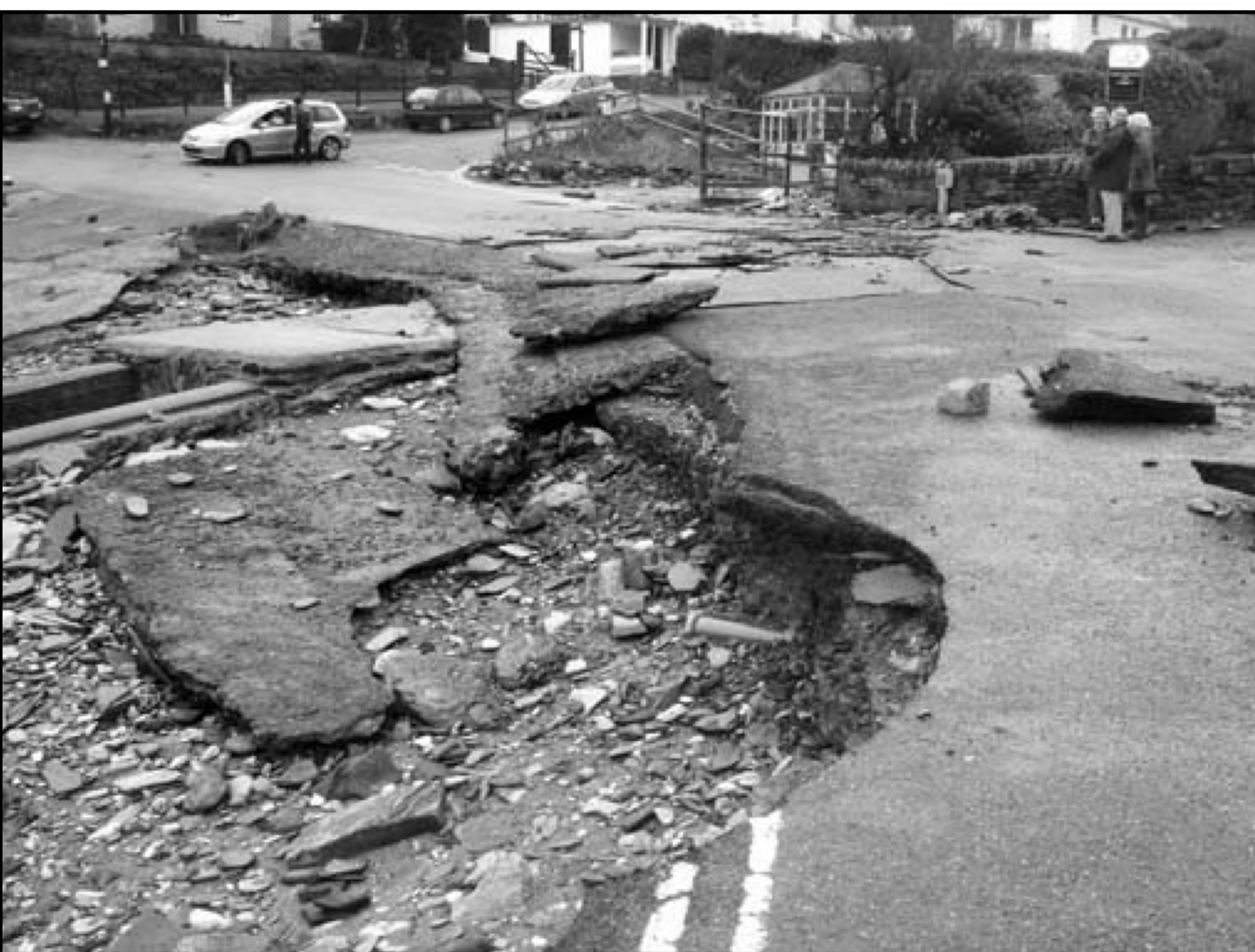
Bob Bulgin's photograph of the storm damaged road at Port Gaverne, taken the morning of Tuesday March 11 th .
